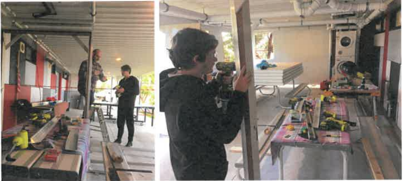
Students have been keen to take on real life construction experiences, with work on the under-croft area being an option.
